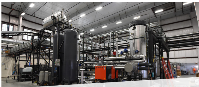
INL's Thermal Energy Distribution System is helping researchers develop the technology to more efficiently use the energy produced by advanced reactors
